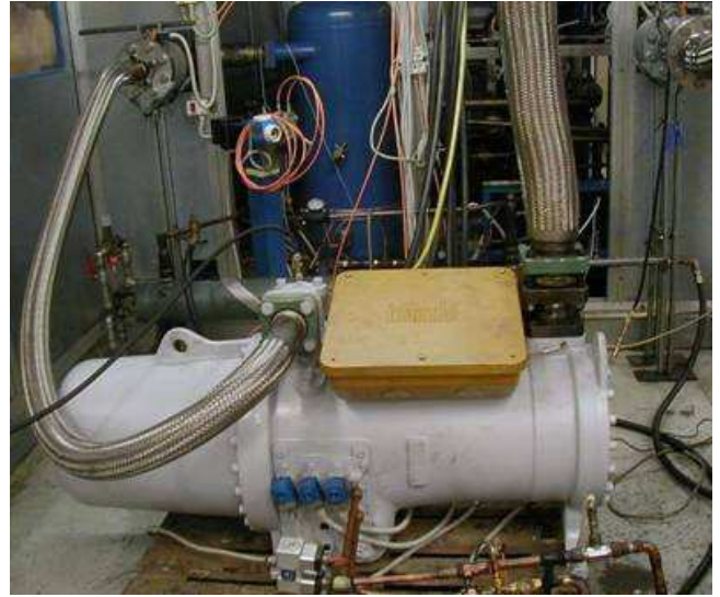
Figure 6 New compressor in the industrial experimental rig
